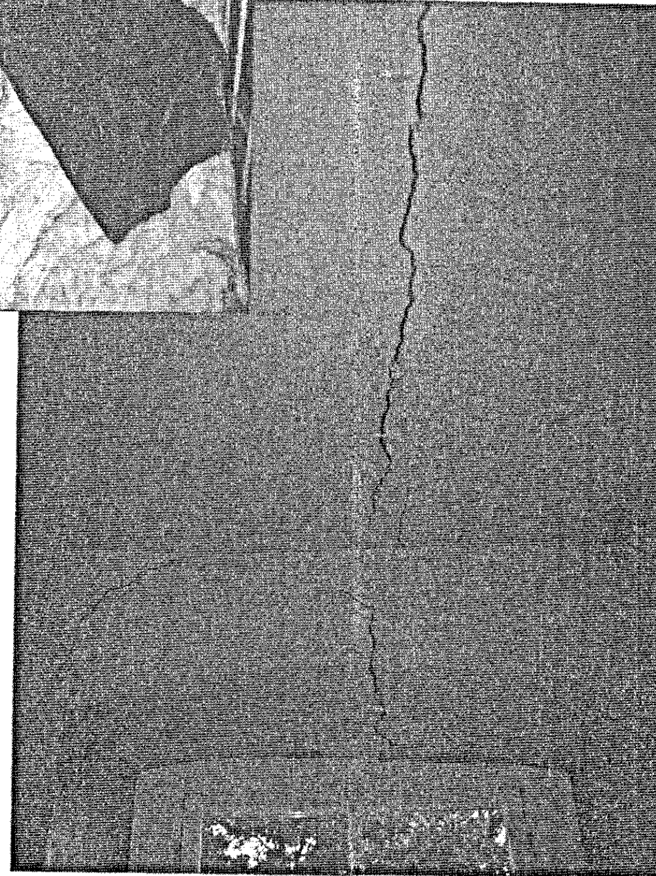
Structural crack through ceiling and window lintols following line of Truss over.
