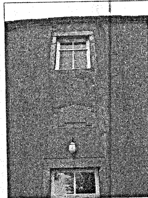
Cracks through external wall
