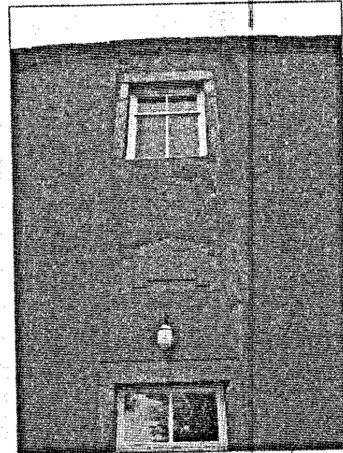
Cracks through external wall
