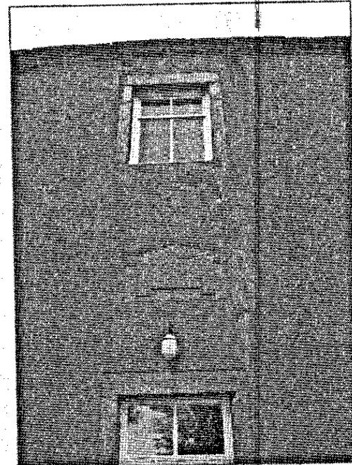
Cracks through external wall
