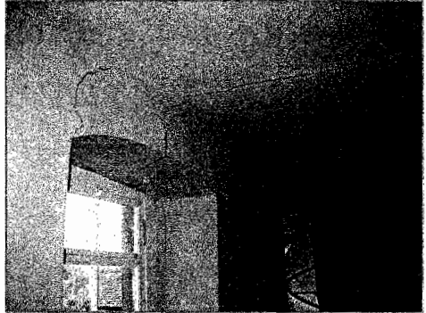
Multiple cracks through central window
